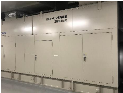
Emergency power generator
