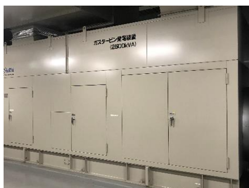
Emergency power generator
