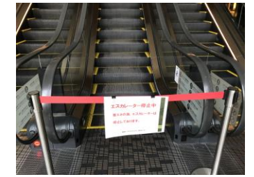
Implemented energy-saving measures with the cooperation of tenants and users (Shinjuku Eastside Square)
